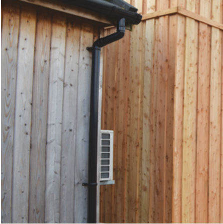
Example of weathered larch cladding next to newly installed, unweathered boards.
